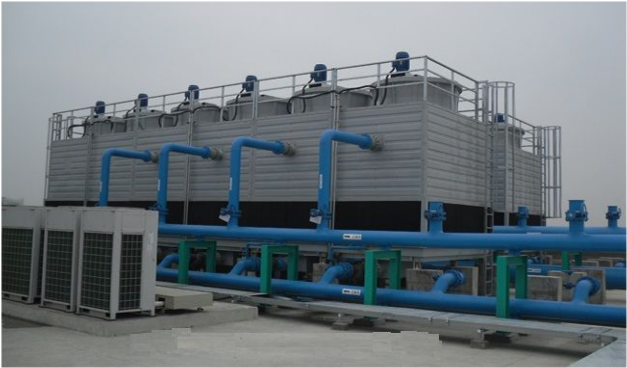
Application of induced draft cooling tower (Reference: pinterest.com )
