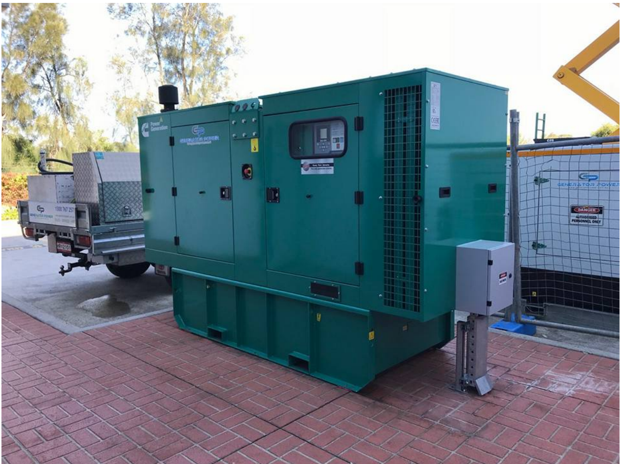
Industrial Diesel Generator (Reference: generatorpower.com )
