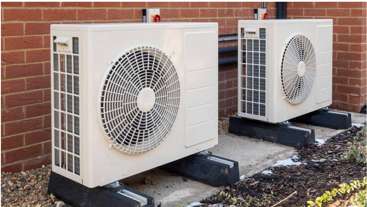
Heat pumps (Reference: howstuffworks.com )
