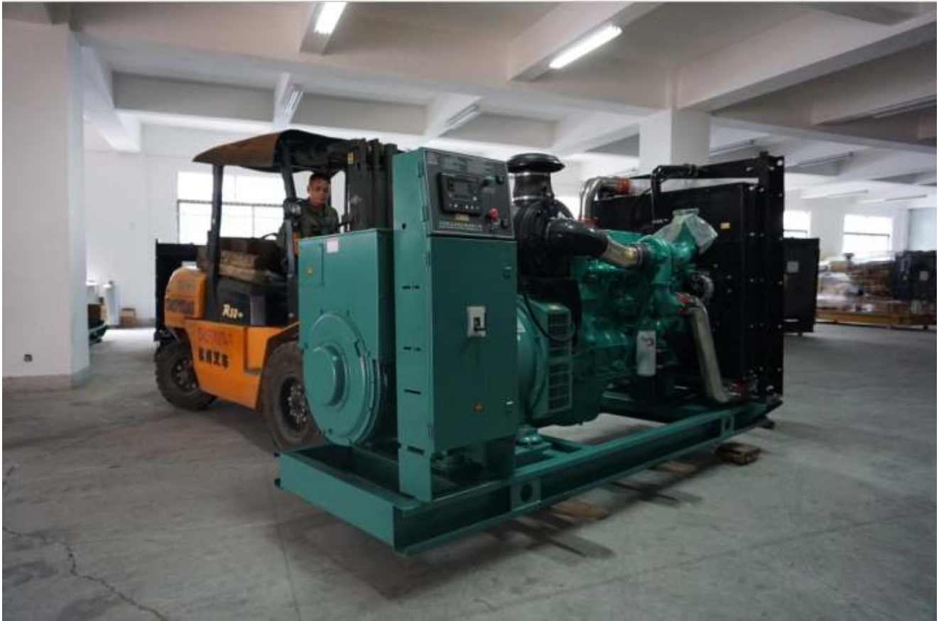
Diesel Generator set (Reference: dieselgeneratortech.com )
